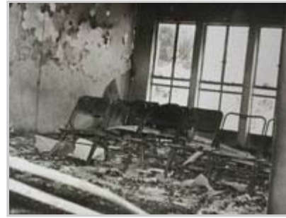
Offices interior after fire, Katlehong.
